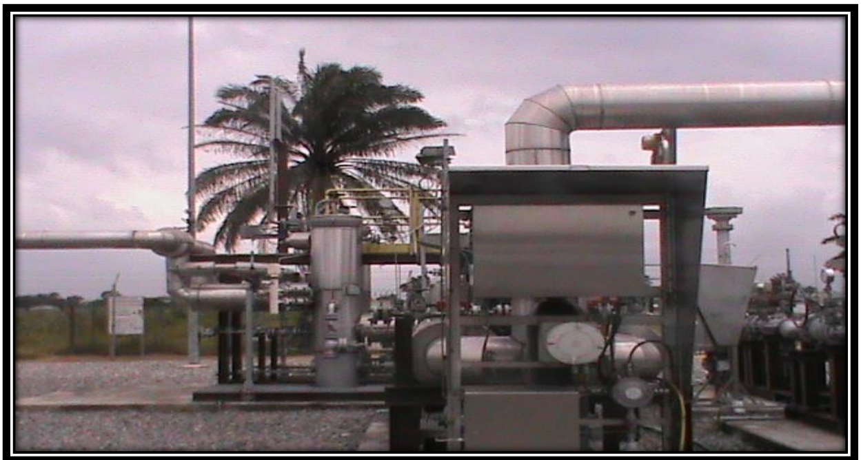
Figure 4. 11: Gas Reduction Section of a Turbine in CS-3
