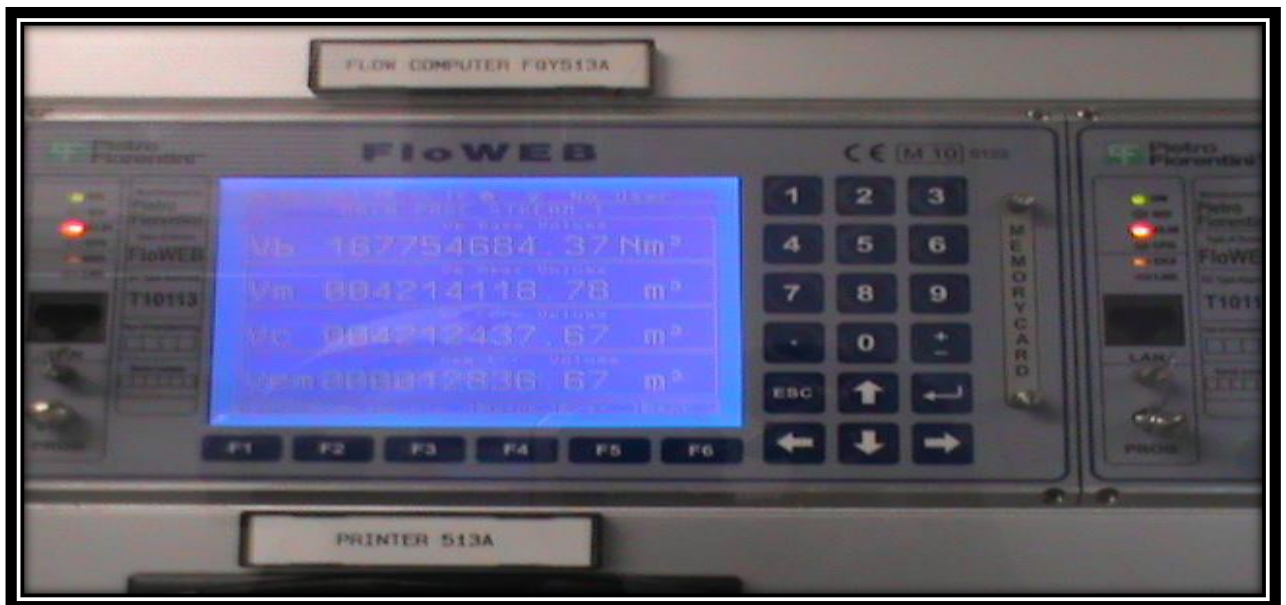
Figure 4. 9: A Section of Floweb Control Panel in the Control Room
