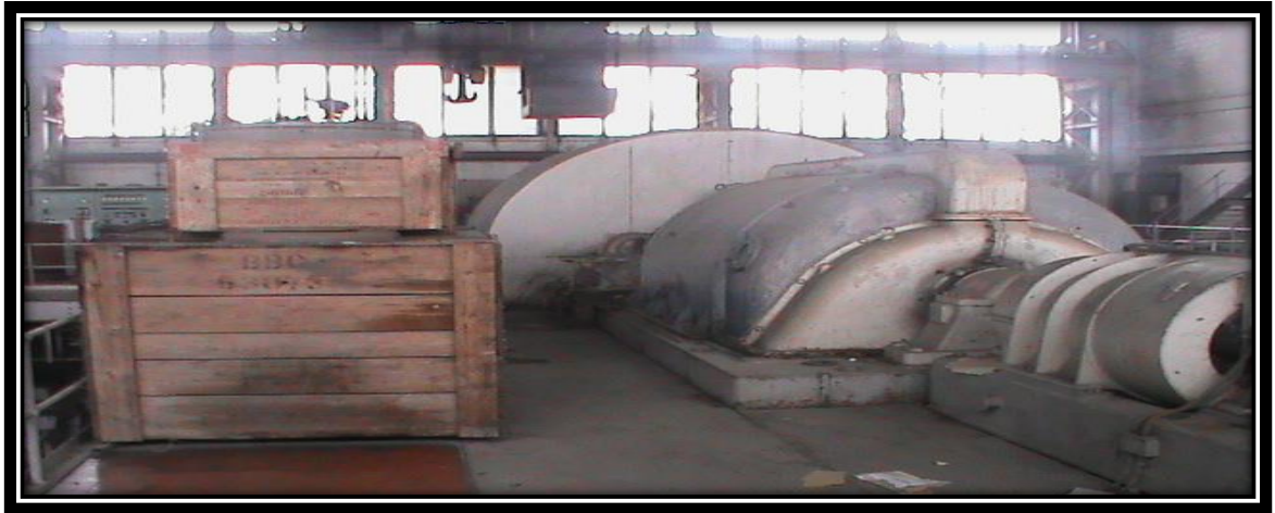
Figure 4. 8: Side View of Gas Turbine in CS-2
