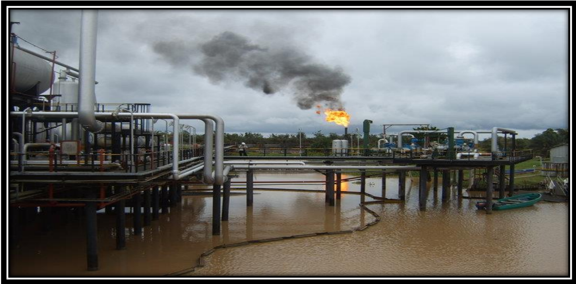
Figure 1. 2: A typical flaring site in the Niger Delta region, Nigeria.
